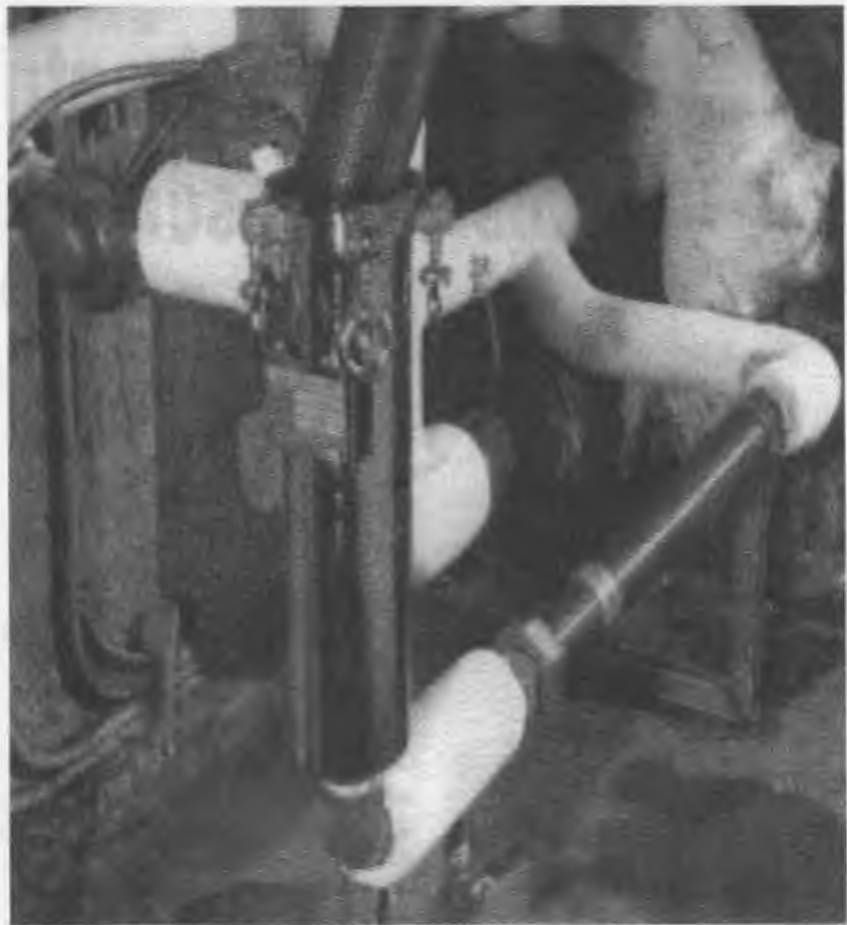
Minerals and impurities remaining in suspension in the water are removed by filtration. Filters are easily replaced.
